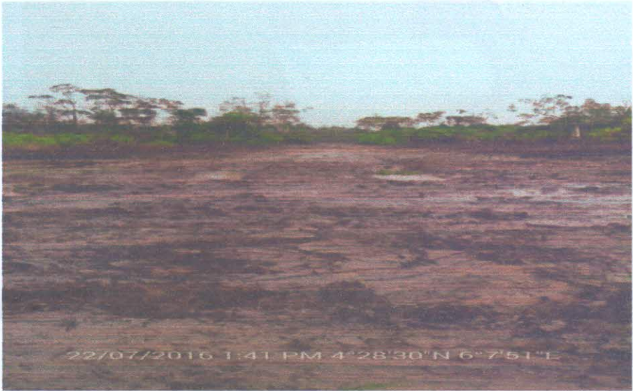
POINT BEFORE REPAIR: fig1
